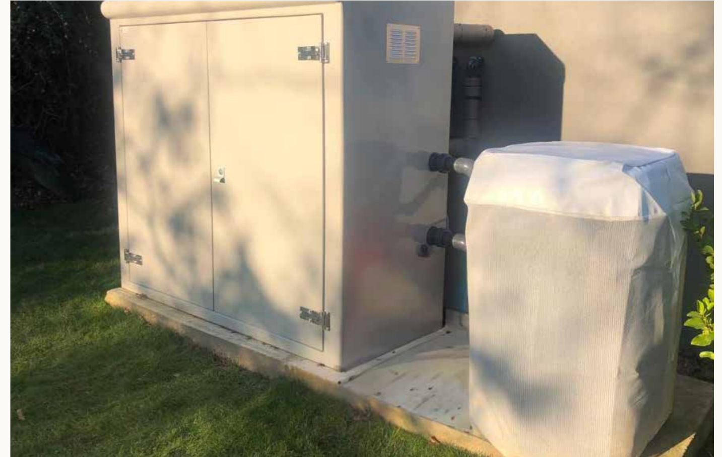
Aqua Technics GRP Filtration Cabinet and Air Source Air Pump
